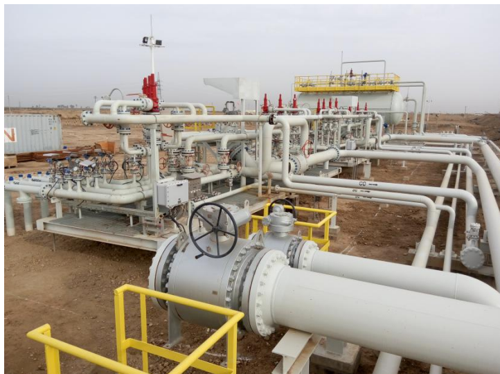
Figure 3. On-site photo of a continuously automatic metering system in a certain oilfield metering station in the Middle East.
